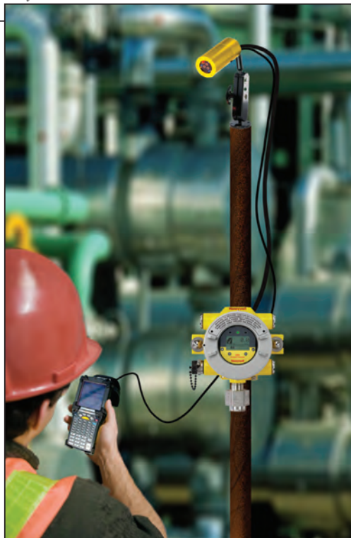
FIGURE 4. Gas detection instrumentation can be made to interface with a handheld communicator, so operators can obtain information from the system or interrogate it, at its point of use. These tools simplify and speed maintenance tasks, so the operator can spend time more productively
